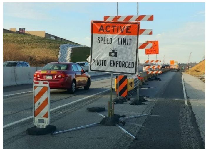
Figure 2. Photo. Advanced sign for a work zone speed safety camera. Source: Pennsylvania Department of Transportation.
