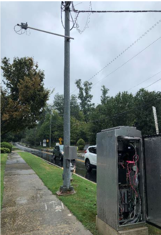
Figure 6: RSU and Cabinet Installation
