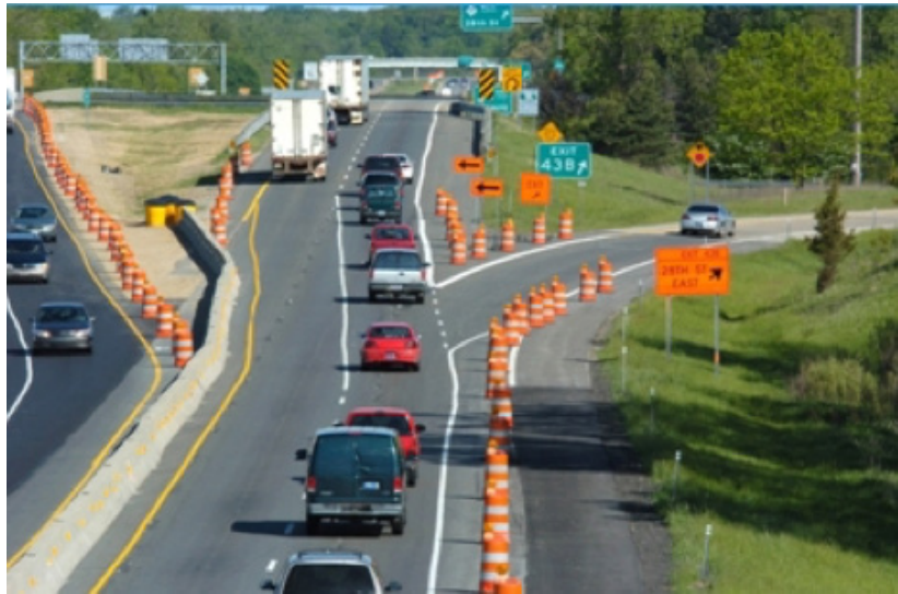
Figure 11. Photo. Traffic directed through a work zone. (23) (Source: Michigan Department of Transportation).
