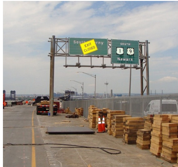
Figure 12. Photo. Center ramps closed to traffic, providing access to construction and emergency vehicles. (24) (Source: NJDOT).
