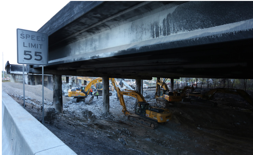
Figure 14. Photo. The I-85 bridge collapse near Atlanta. (27) (Source: GDOT).
