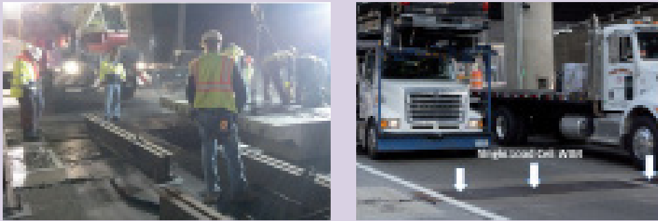
Figure 1. Pre- and post-installation of a WIM scale by NYCDOT (photos by NYCDOT)
