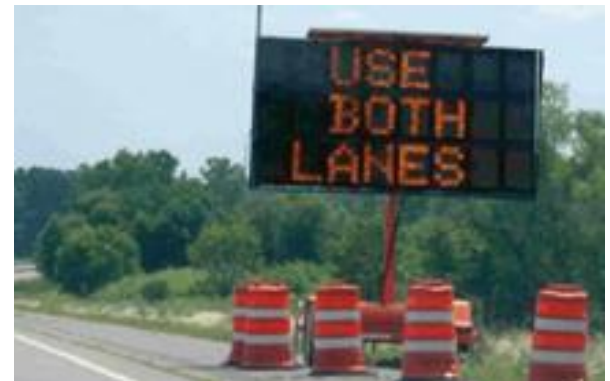
Dynamic Late Merge system in a Minnesota work zone.
