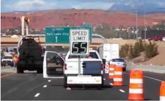
Example of a portable regulatory variable speed limit sign used in a Utah work zone.
