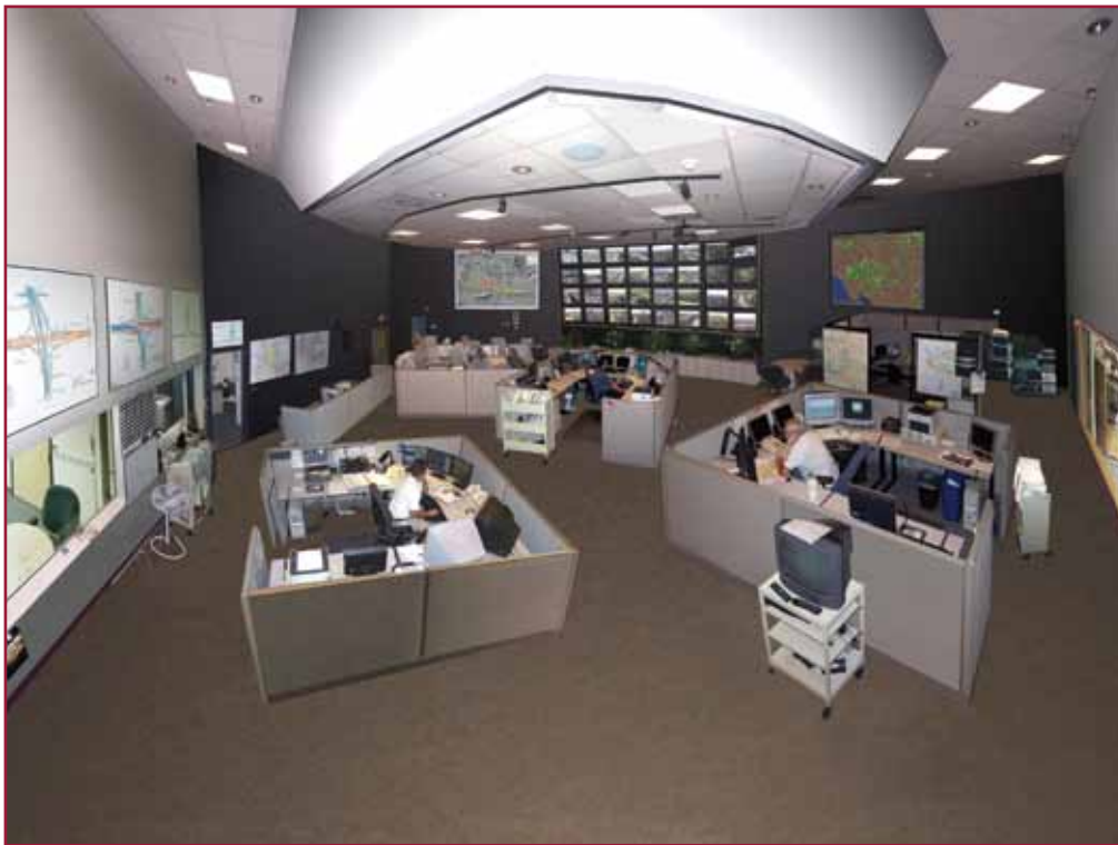
Arizona Traffic Operations Center
