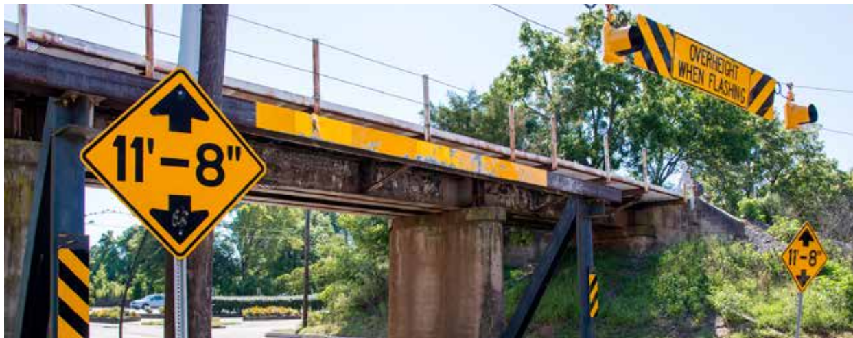
The Gregson Street Bridge with the previous overheight detection and warning system. Source: Washuotaku, Wikimedia Commons, licensed under the Creative Commons Attribution-Share Alike 4.0 International license.
