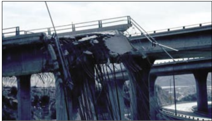
Figure 2-3. Damaged freeway-to-freeway ramp after Northridge earthquake. (Source: U.S. Department of Transportation 7 )
