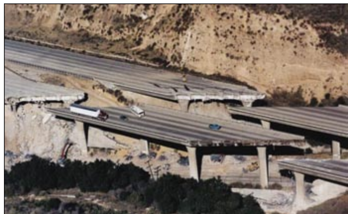
Figure 2-4. Damaged freeway mainline section after earthquake. (Source: U.S. Department of Transportation 7 )
