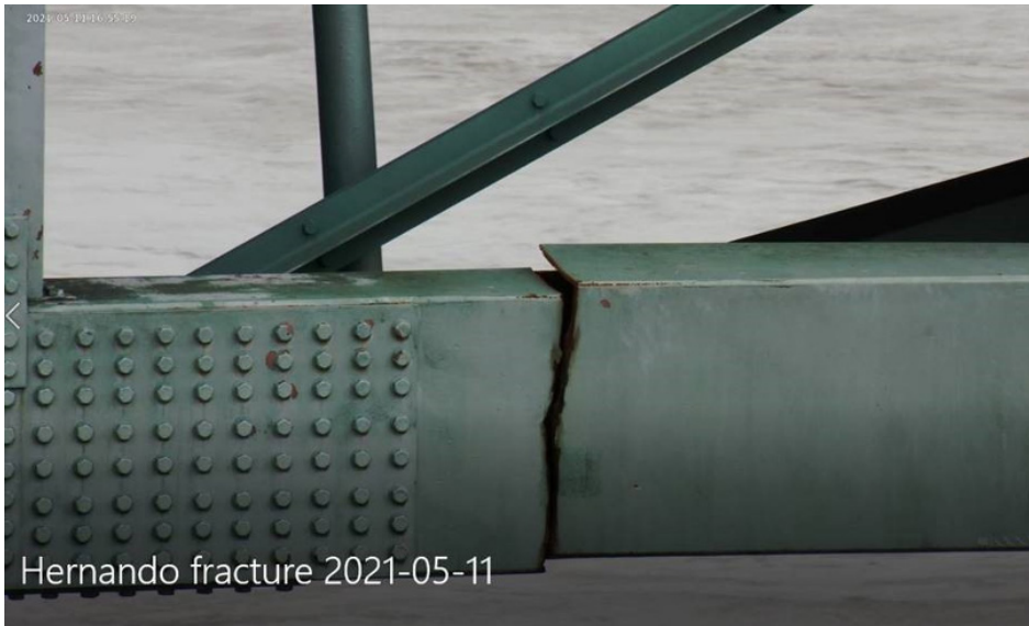
Figure 1. Photo. Tennessee Department of Transportation bridge cracked beam. Source: Tennessee DOT Library. (tn.gov)
