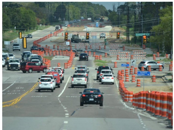
Figure 1. Flexibility in addressing unforeseen conditions in work zones is often needed to improve safety.
