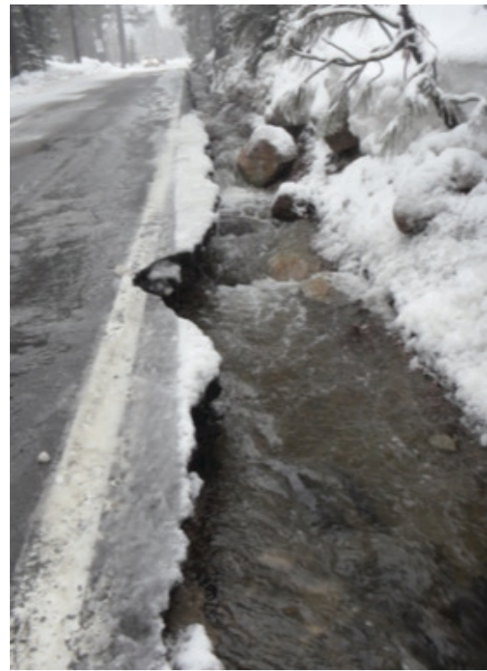
Figure 5: Impact of flooding on Truckee roadways. (Source: Town of Truckee, CA)
