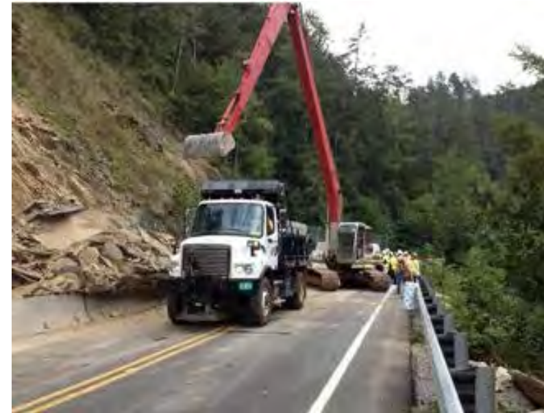
Landslide from heavy rain in August 2013. Source: TN DOT
